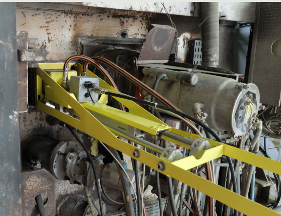
→ Pyroscan installed close to the kiln burner
